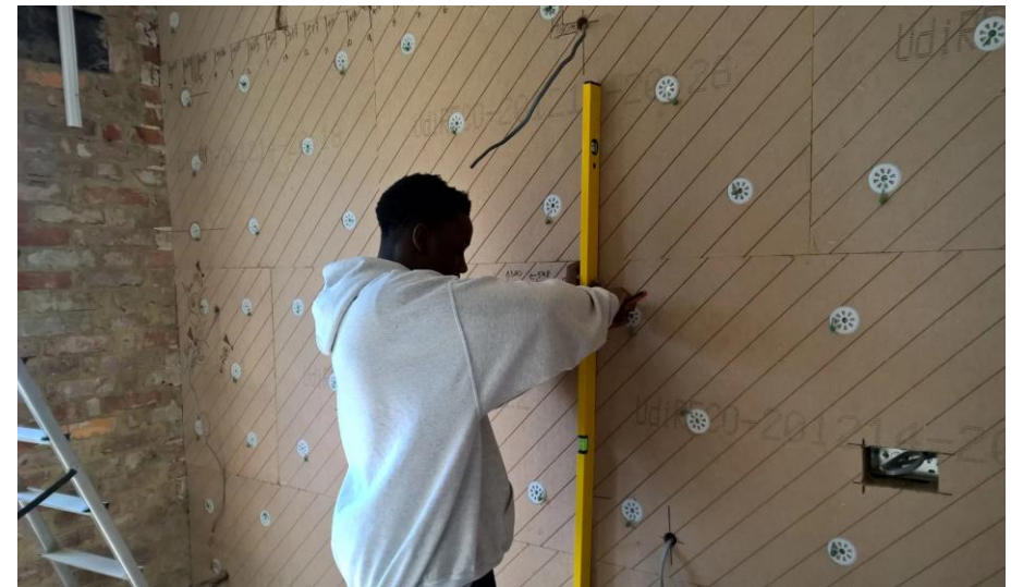
Installation of wood fibre insulation boards internally (Sources Back to Earth & ASBP)
